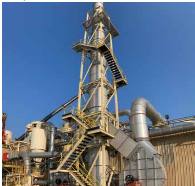
Originally designed as a stand alone stainless steel stack, this project required innovative thinking to keep it on budget in a volatile steel pricing market.
