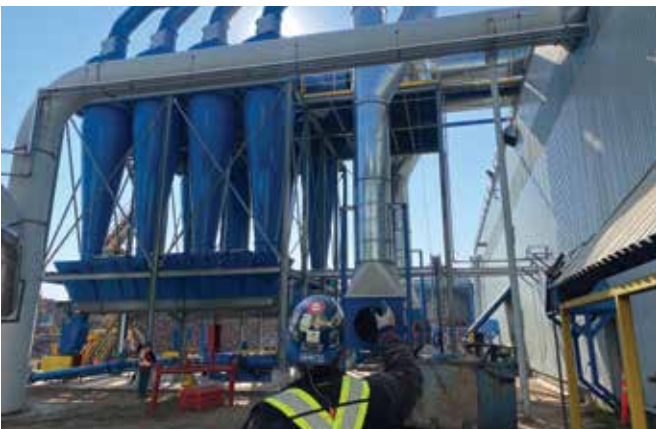
A VETS Sheet Metal team member is dwarfed by the size of this super efficient multi-cone cyclone.
