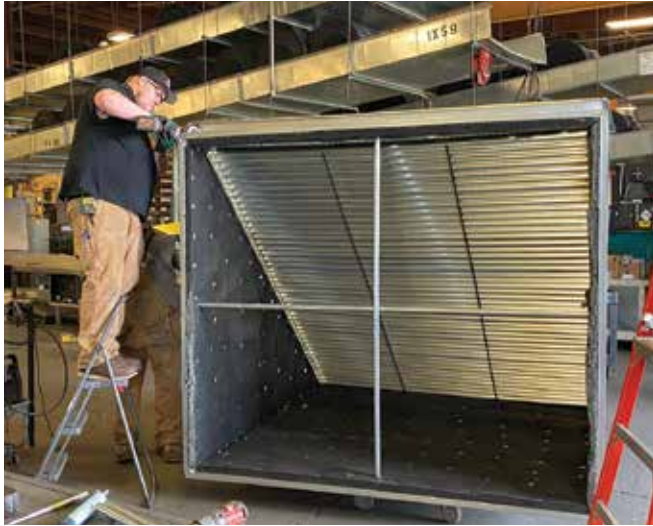
Sheet metal work for the Summit Building at MacDonald-Miller prefabrication shop in Seattle • Photo by Rylan MacCay
